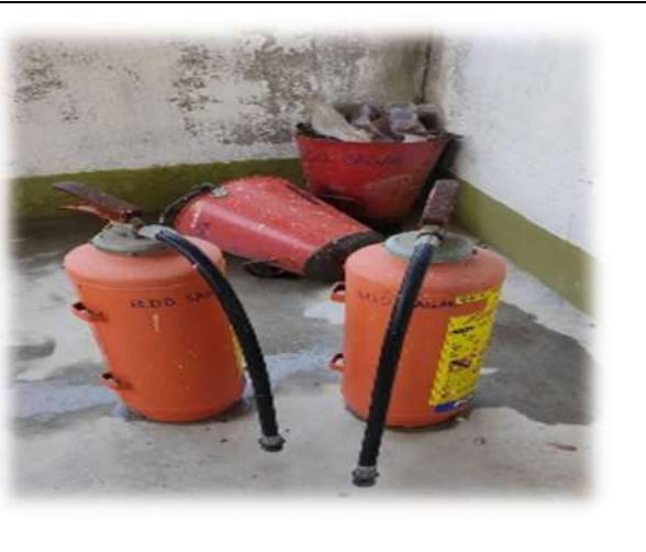
Fire Extinguishers are not placed properly
